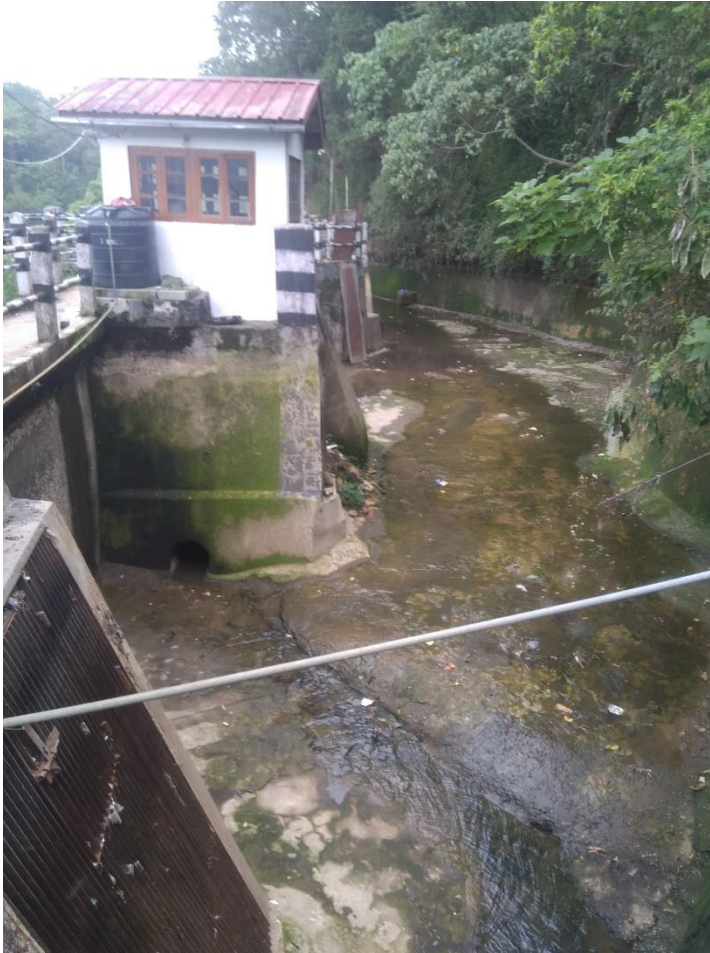
Figure 4 In-take Gate of Sonapani Mini Hydel Project at Umshyrpi Stream
