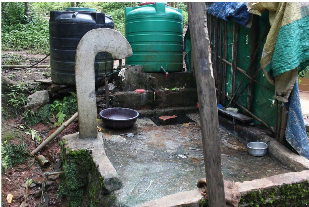
Figure 4 Non-functioning Water Pump on Project Site
