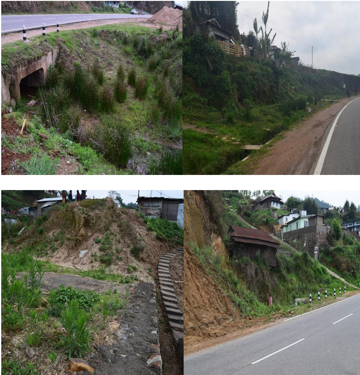
Figure 4 Shows the dumping of soil near paddy field and concern of mud slide near household area.
