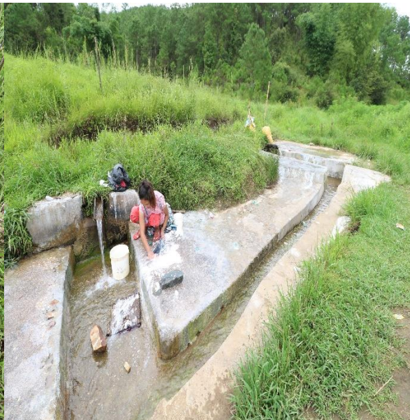
iv. Loss of washing platform
