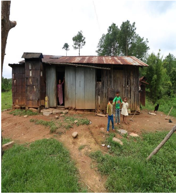
v. Loss of structure
