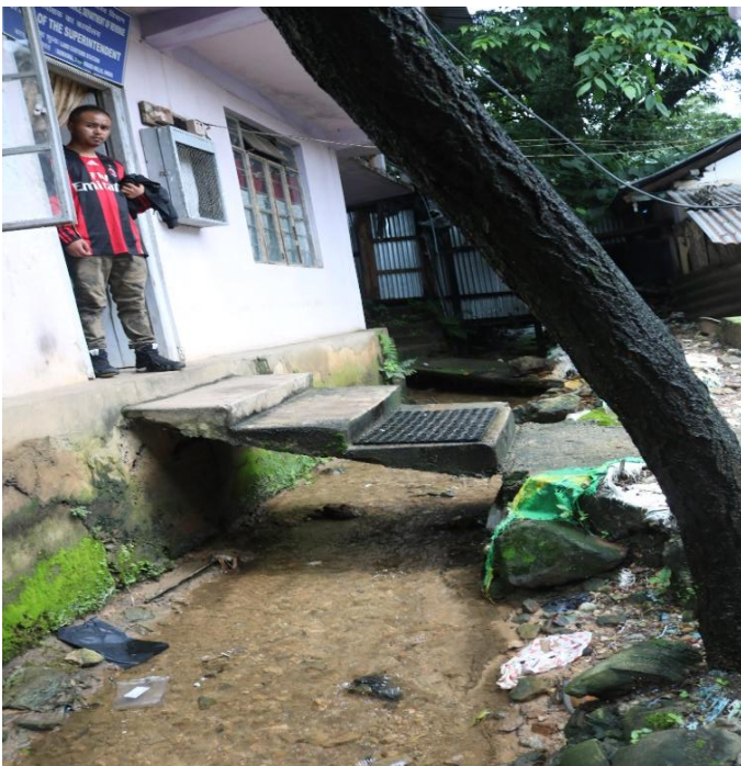
v. Lack of proper drainage/ without slab
